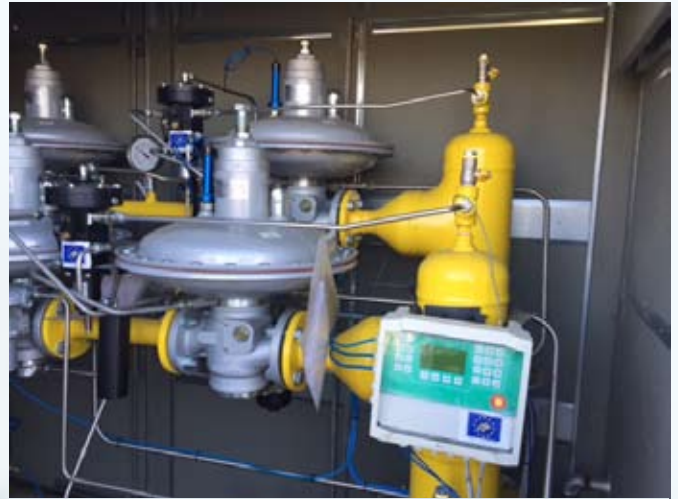
fig.7: FIO 2.0 device inside a PRMS
