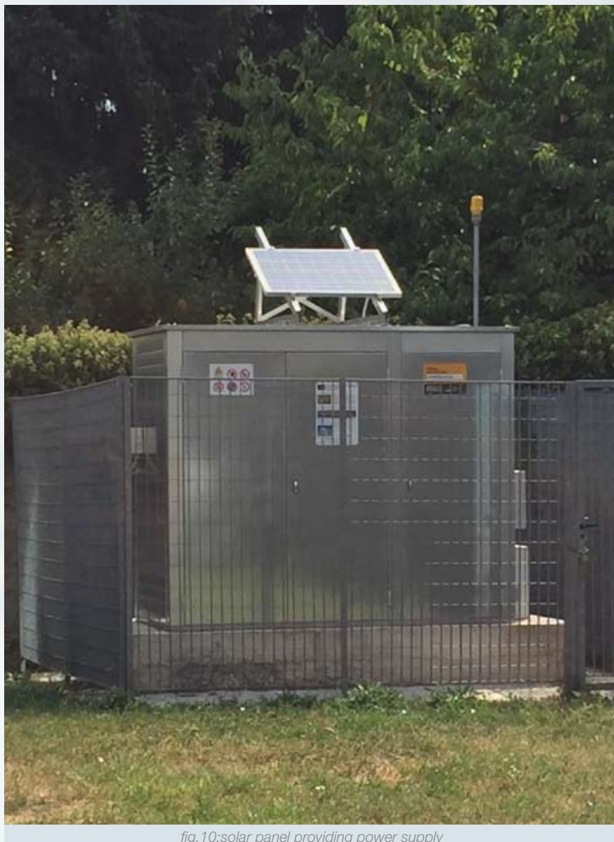
fig.10:solar panel providing power supply
