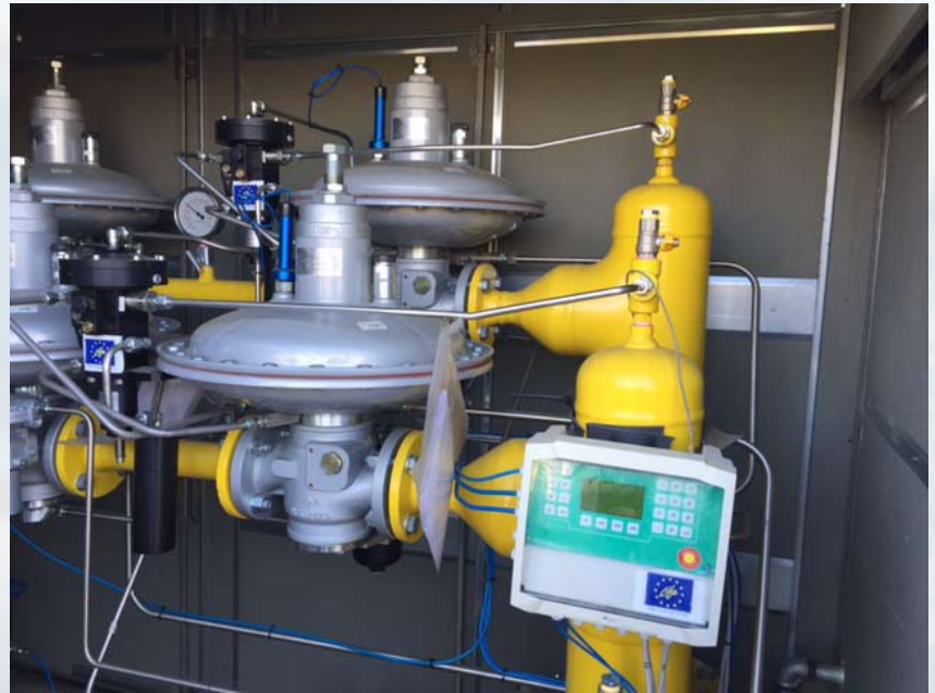
fig.5: FIO 2.0 device inside a PRMS
